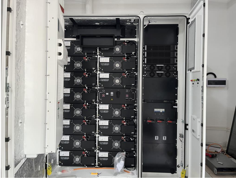
铭牌, 电池柜 (label, Battery cabinet) -6
