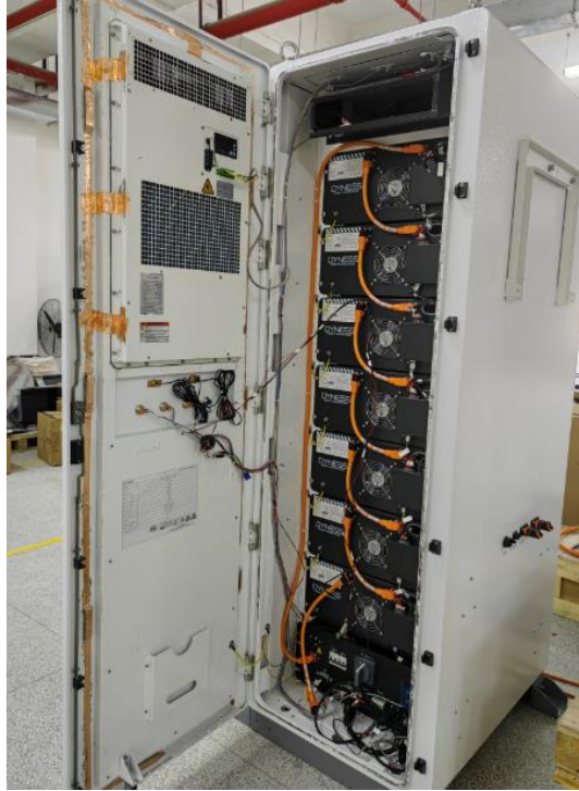
铭牌, 电池柜 (label, Battery cabinet) -6
